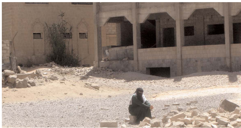
Many schools in Yemen, such as Al-Mujamma' Al-Tarbawi in Bab Al-Yemen (pictured), were never finished or were poorly built and now in danger of collapsing.
