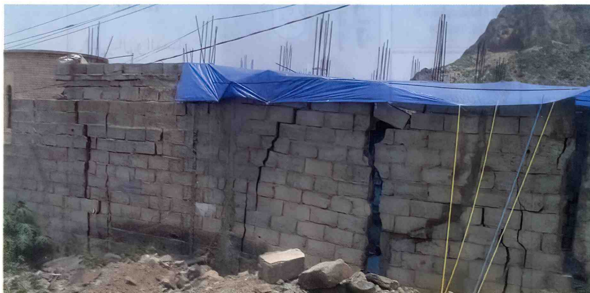
Houses nearby effected with discernable cracks
